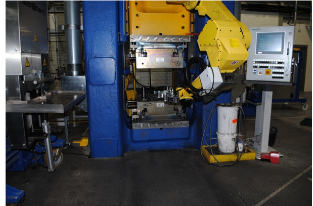
Figure 16. Fanuc M710 robot mounted inverted on Gantry.
